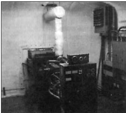
Figure 7. WI101509 engine generator enclosure including 100 kV generator set, skid base, foam insulation, lighting, fire alarm, lowers, fuel tank, etc.
